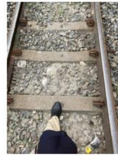
Gambar V. 3 Mud Pumping di Area Bekas Genangan Air
