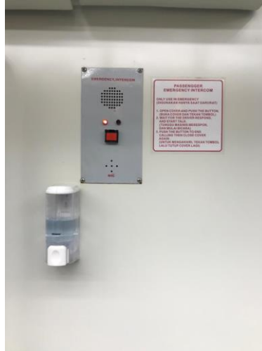
Gambar II.12 Passenger Emergency Intercom LRT Sumatera Selatan
